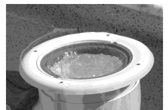
Additional flow after restricting other returns
